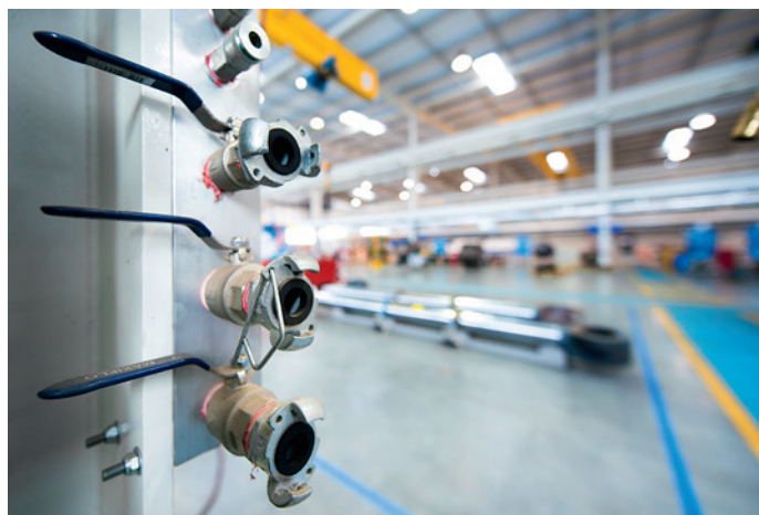
With seven manifold outlets installed at different points throughout the facility, compressed air is highly accessible when and where required.
